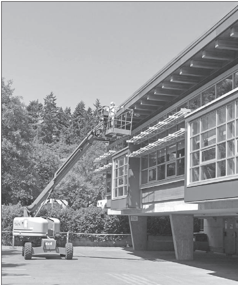
11:57 am Colin Lamb paints the back side of the 12,500-square-foot Salt Spring Public Library building, which was opened in 2012.
