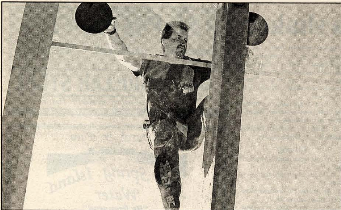
TOP OF THE WORLD: Troy Kaye of Gulf Island Glass works with Kevan Andrews, Phil Gregson and Roy Cronin to install a new piece of glass Monday, covering the outdoor dining area at Moby's Pub.
